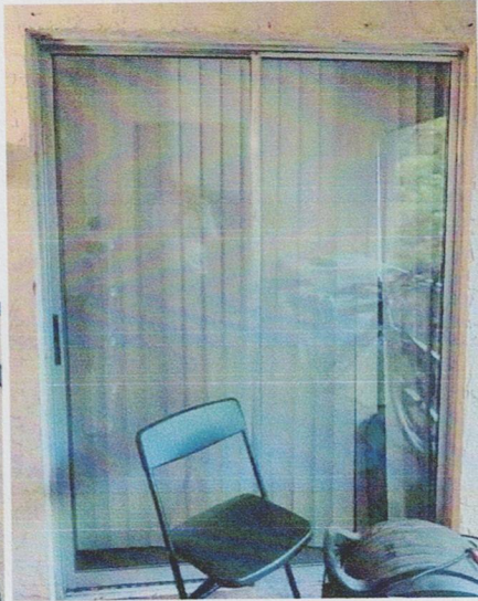
Unprotected glazed entry door
