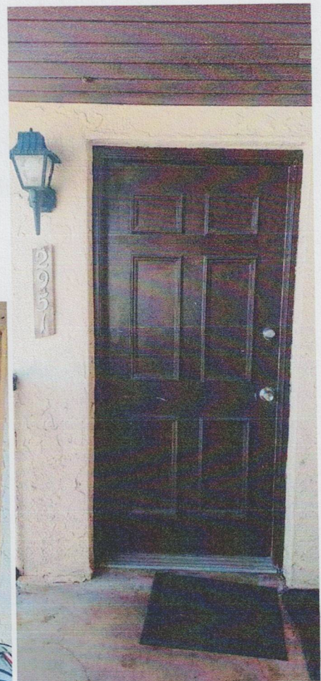
Unprotected non-glazed entry door
