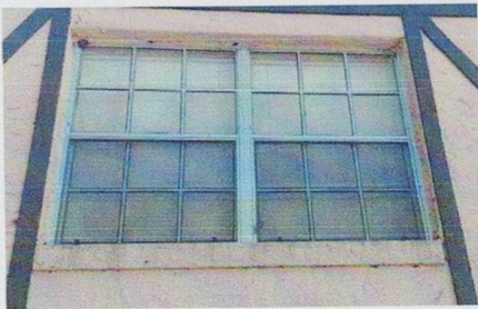
Unprotected glazed opening
